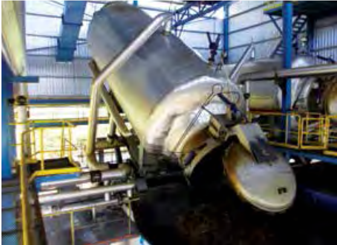
The new tilting steriliser installed in Segaria Palm Oil Mill in Sabah
