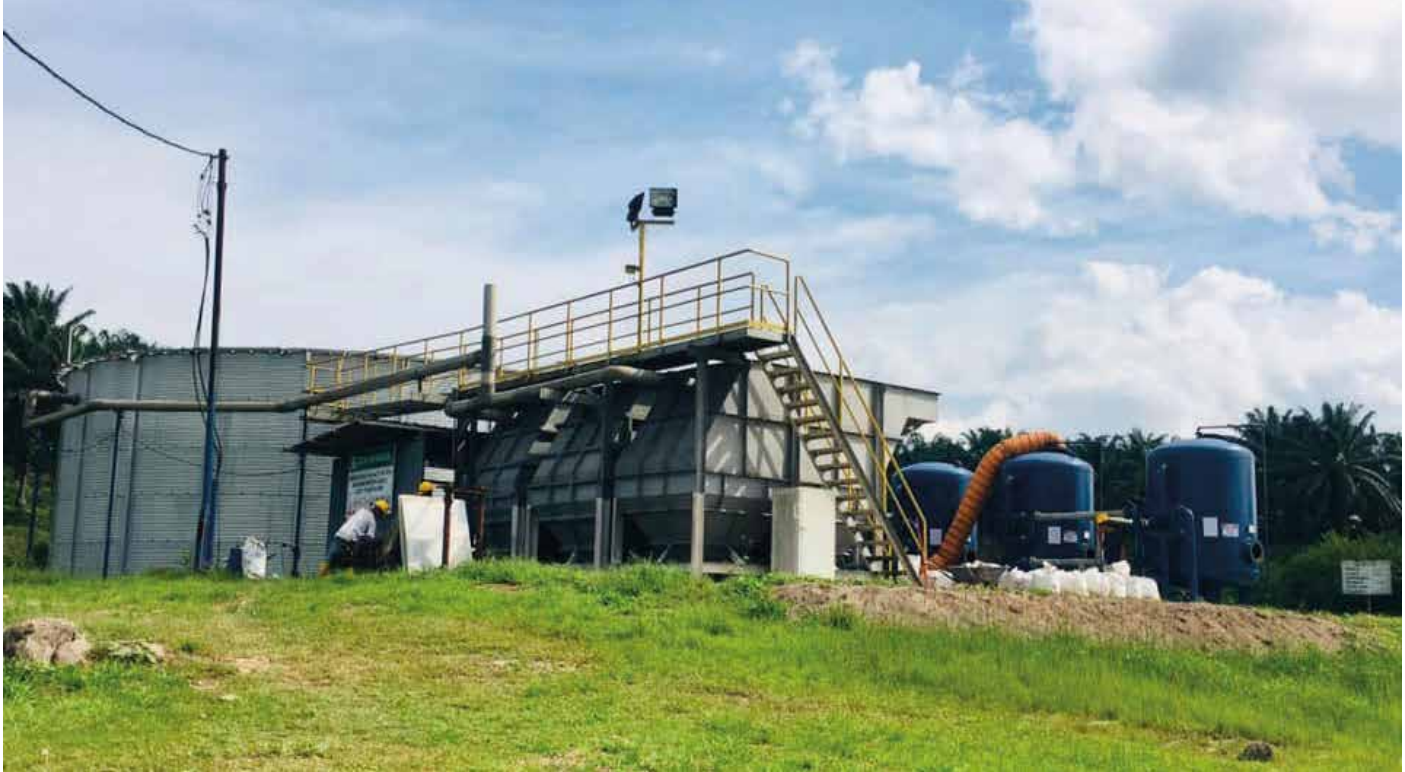
Tertiary Plant for Effluent Treatment at Tawai Palm Oil Mill, Telupid, Sabah
